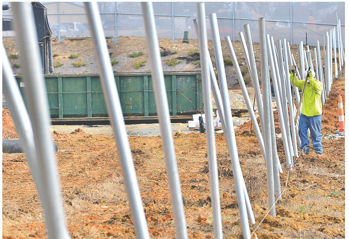
One down, 100 to go! That's probably what this worker is thinking as he installs fence poles on the Moutaire Poultry property. The worker was lucky, we guess, all the holes were dug mechanically, using a power auger. But some old-fashioned work had to be added to the holes to make sure they were at the correct height. He was spotted by Chatham News+Record photographer Jeff Davis on East Raleigh Street in Siler City last week. (Staff photo by Jeff Davis)
